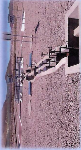
CONST. SIST. ALCANT.SANIT. LA LAJA (MORO MORO)
